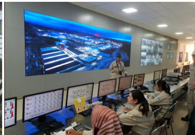
RKEF Control Room
