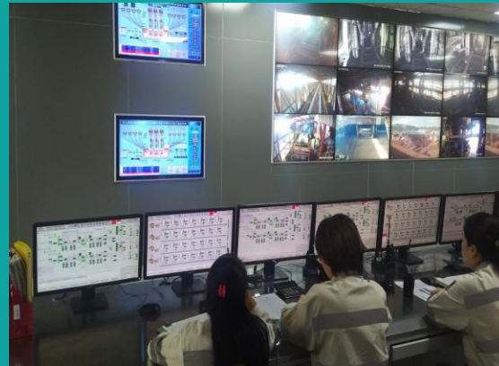
RKEF Control Room
