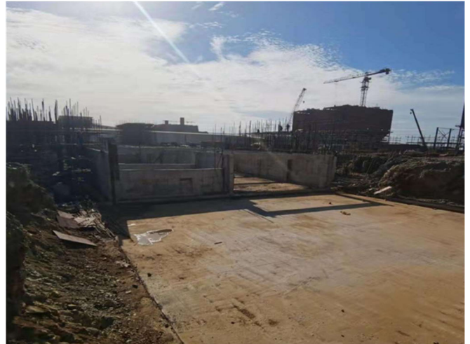
Slag flushing circulation pond
