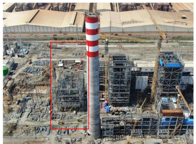
Aerial view of power plant
